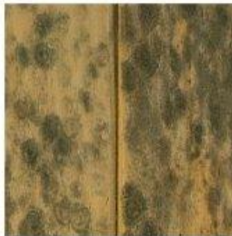
Pressure treated timber that mould has been allowed to grow. The difference between the treatments salts and mould is quite clear.
